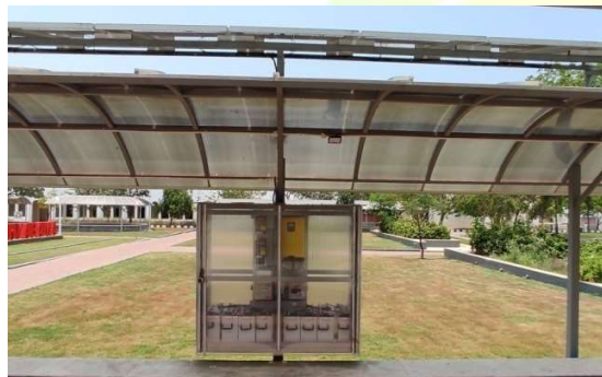
Figure 46: Solar panels with controller
