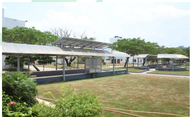
Figure 18: Solar panels with controller
