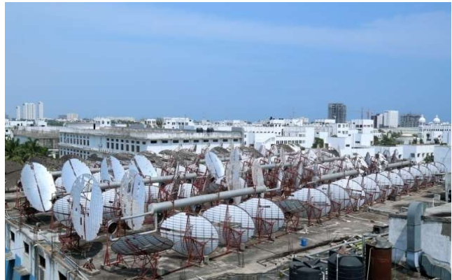
Figure 14: Solar cells on roof top
