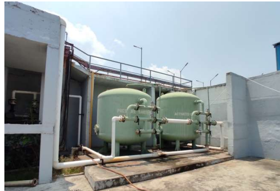
Figure 8: Water treatment unit
